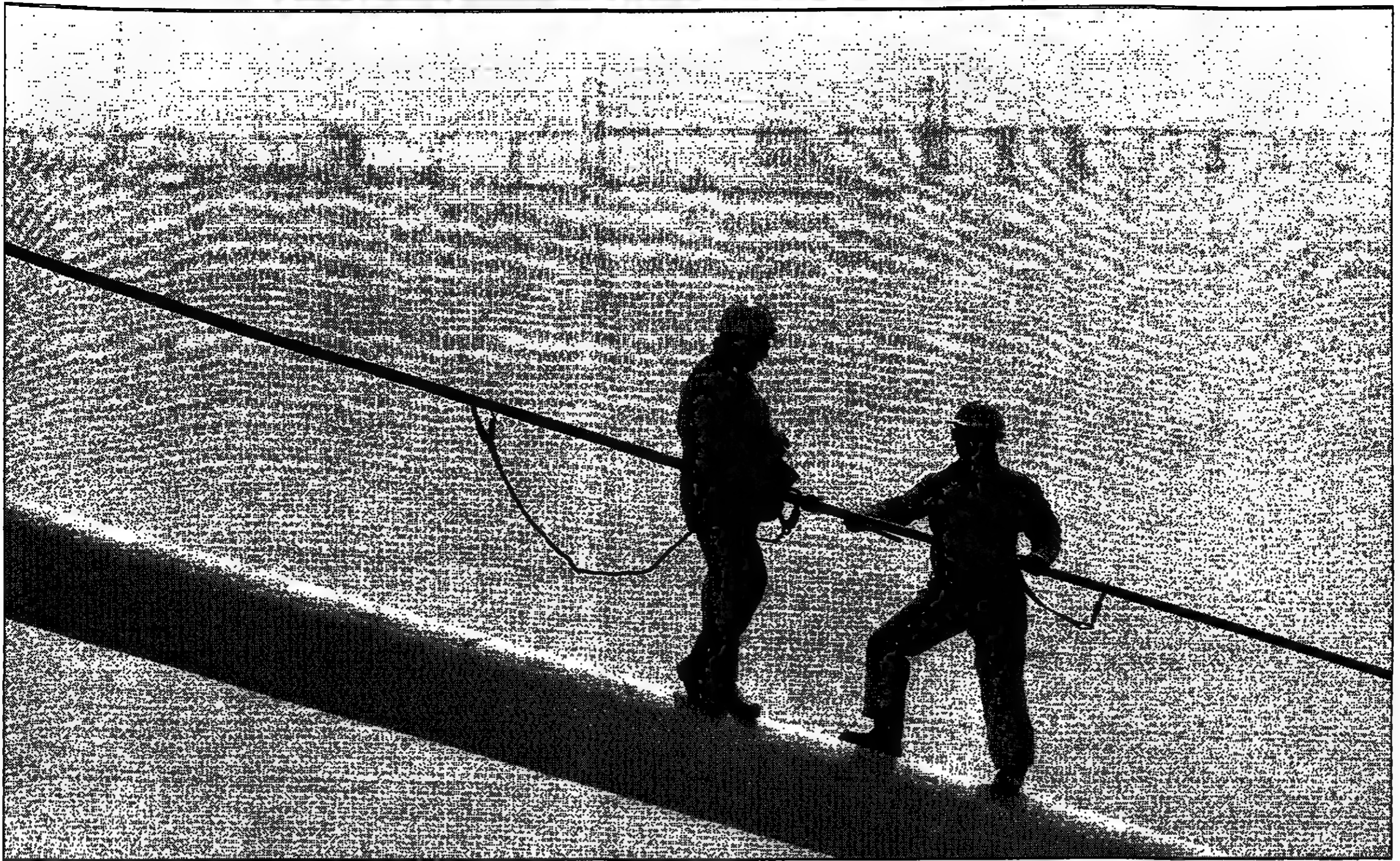
A job with a view... painters Dave Whatmore and Jed Needs at work on the bridge. In the background the Second Severn Crossing which opened this week
